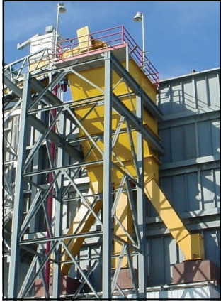
Coal Chute Lined with 10 Gauge CRODON Standard
